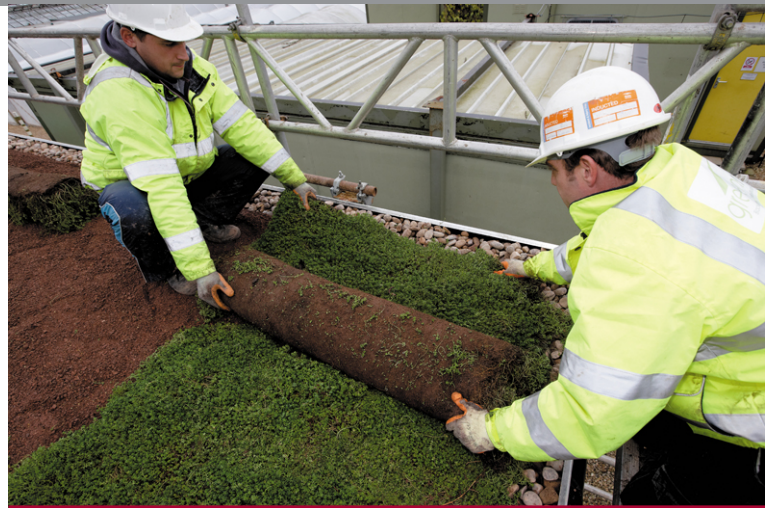
The multi-layer VerdiRoof system was installed over FDT's Rhenofol single ply waterproof membrane.
