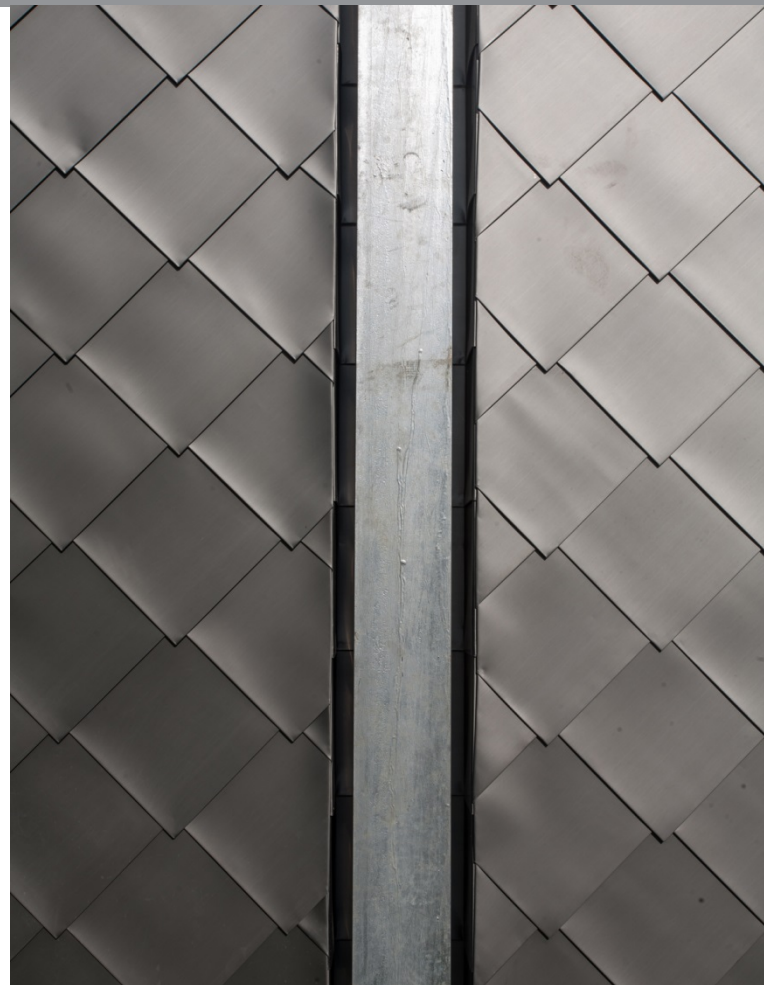
'A very honest, natural coloured material' NedZink NOVA shingles trim the dolphins. Photo © Baca Architects
