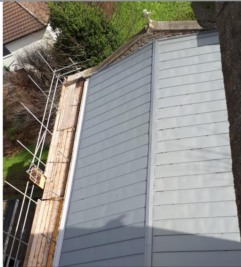
A zinc coating, elZinc Slate, was chosen to create a ‘like-for-like’ finish on the pitched roof.
