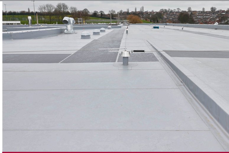
SIG Design & Technology's new flat roof package is a part of the ongoing construction works.
