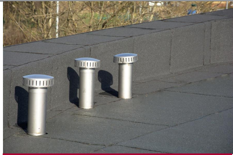
A crucial phase of the work was the correct detailing of the junctions with the flat roof.
