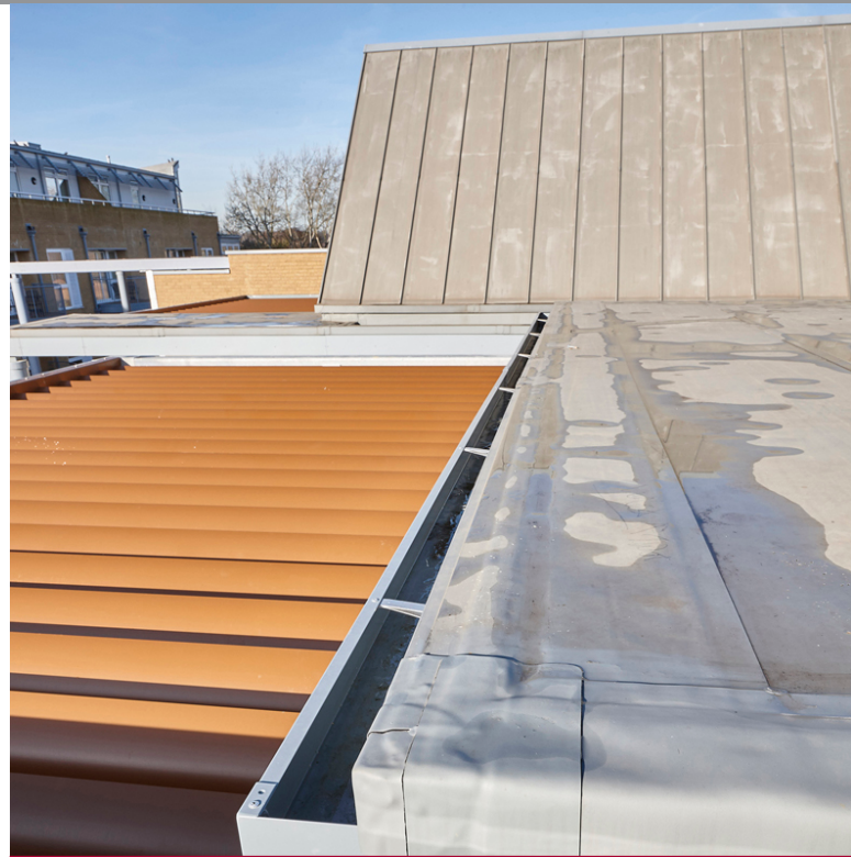
With the project spanning a total of 11,931m 2 , the overall scale of the project was large and meeting programme schedules for the following trades demanding.
