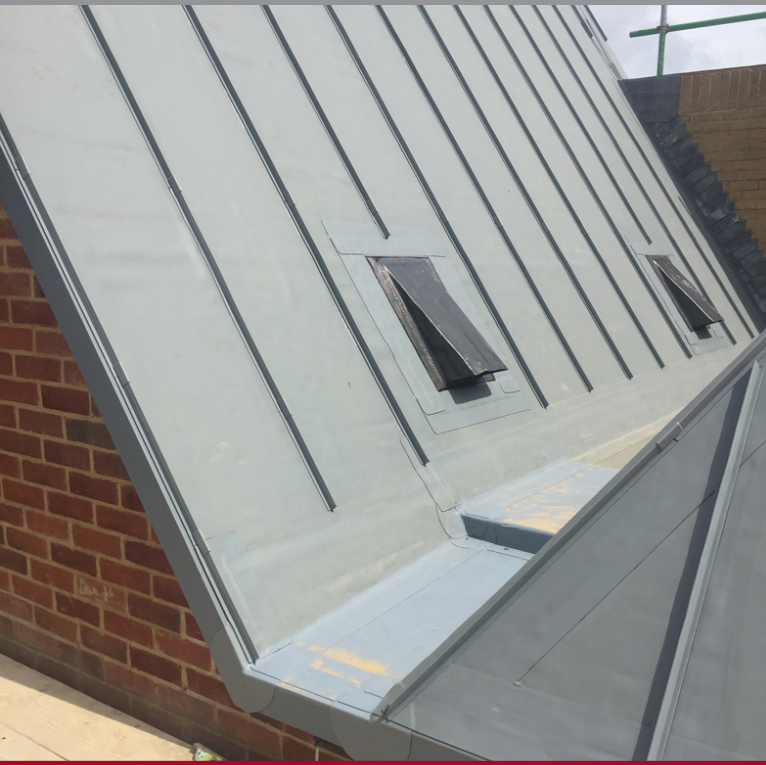
Four distinct types of roof areas demanded that the installation team drew upon all their knowledge skills and experience.
