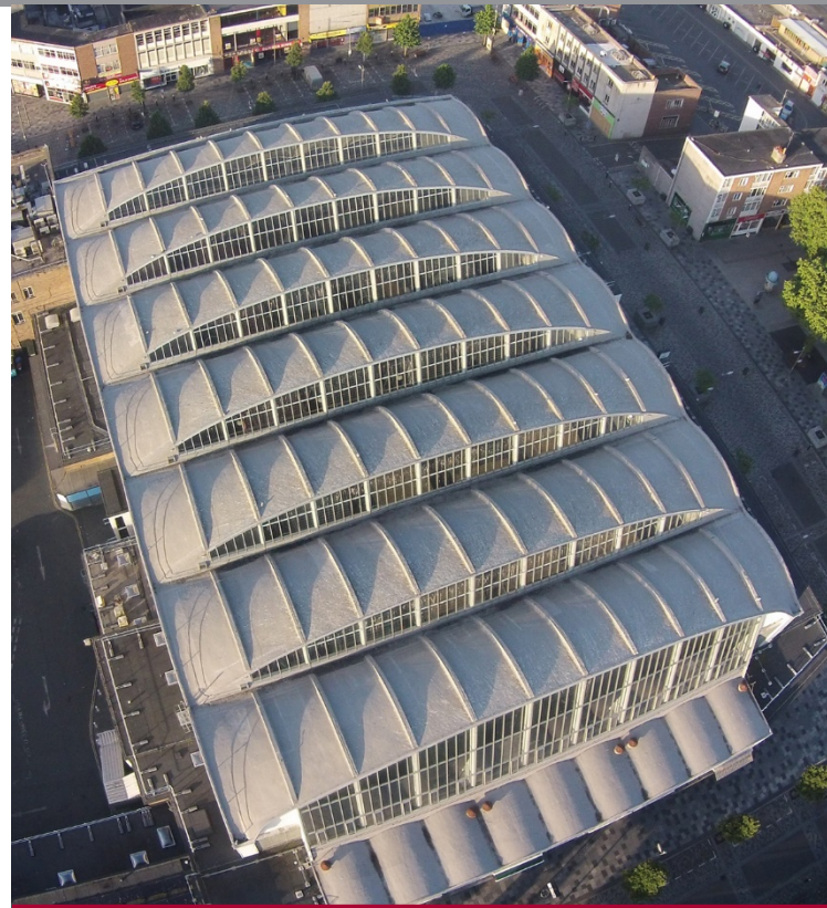
Hydrostop AH+ provided the perfect solutions, allowing traders to continue "business as usual" while roofing work was in progress
