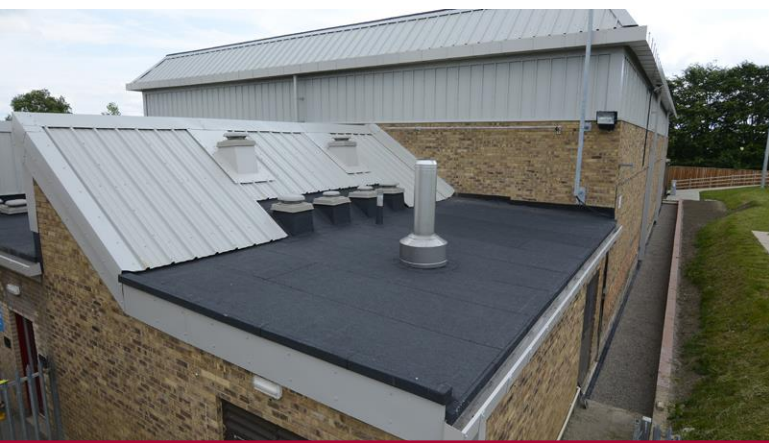
The Gym Hall and Changing Rooms were completely refurbished with the SIGNature bituminous torch-on system and Steadman's composite panels
