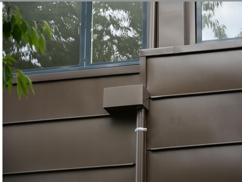
It was necessary for the horizontal bands to track right round the terrace front and back
