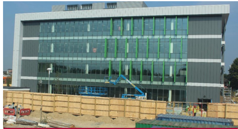
The Hydrostop AH+ system was applied over a concrete substrate with a bituminous vapour control layer.
