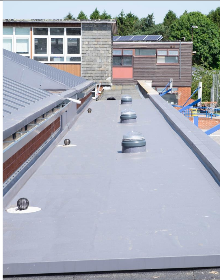
The bonded warm roof construction to both flat and pitched (pyramid) roof areas was waterproofed using IKO's bonded Armourplan PSG membrane
