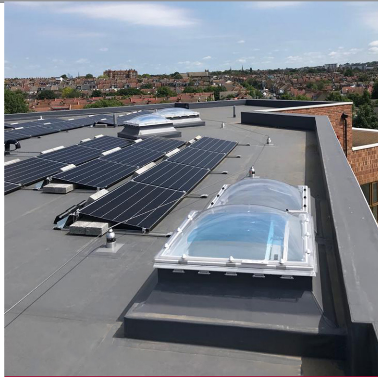
Armourplan PSG system was chosen to waterproof the main roof area complete with rooflights and solar panels.
