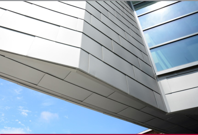
Non-centered shingle set-out creates a less zig-zag facade effect. Photo Terence Smith Photography
