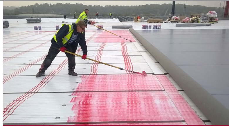
IKO Polymeric manufactured its Armourplan PVC single ply membrane in bespoke rolls to reduce waste and installation time for this project.
