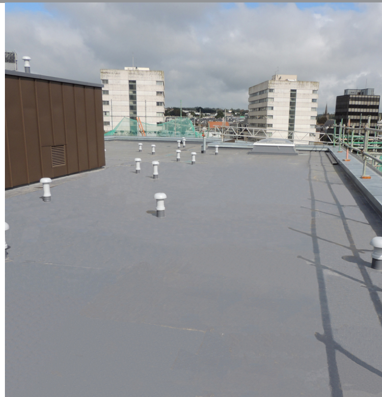
Armourplan PSG system was chosen to waterproof 800 m 2 of the main roof area.
